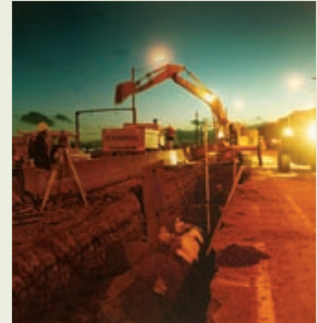
The ‘ten-fifty’ project in the late 1970s greatly increased the supply capacity of the pipeline from Wainuiomata to Wellington.
