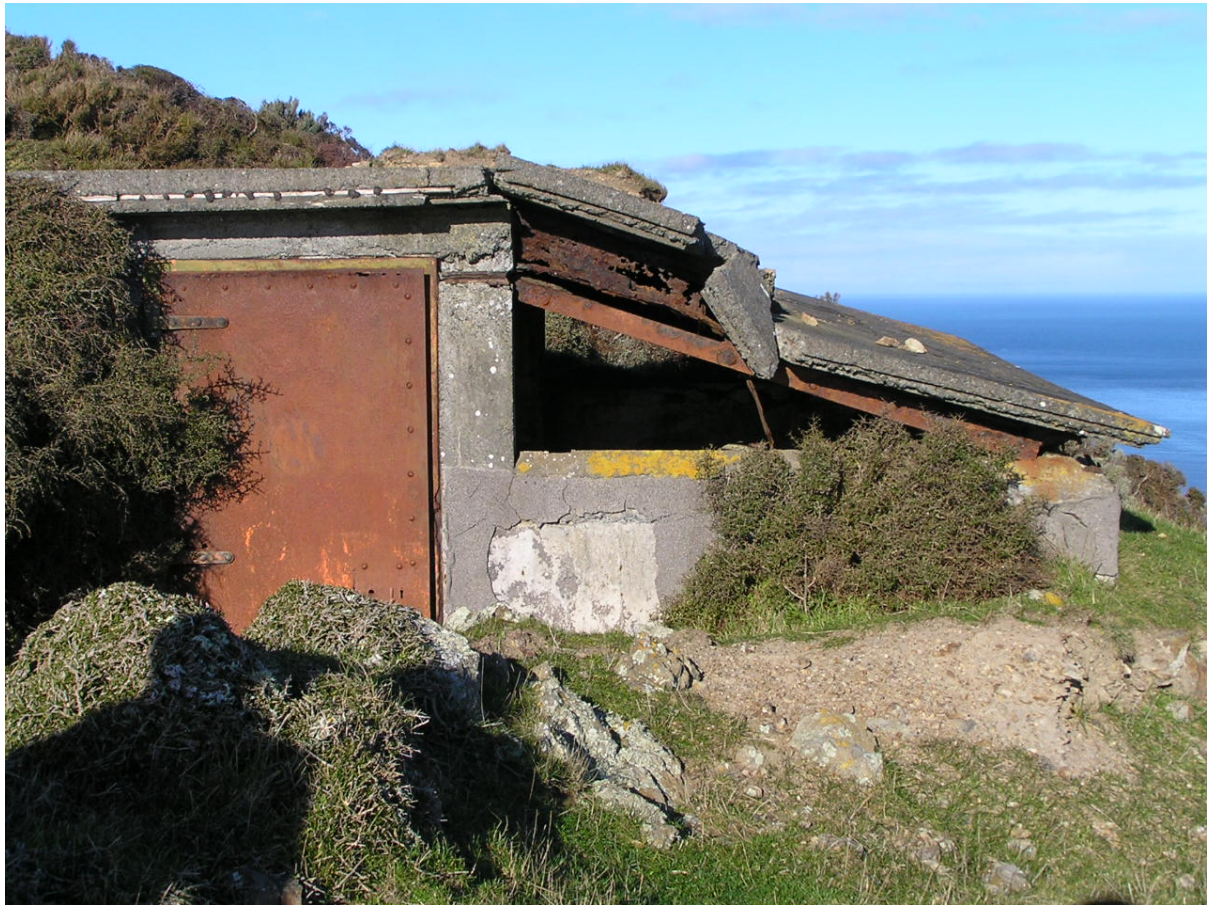
Observation bunkers in need of stabilising before the public can access the site
