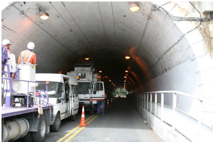
Seatoun tunnel from Ferry road – showing existing overhead running wire with some splices
