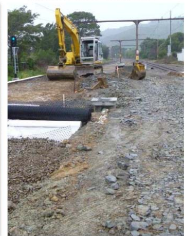
Hardfill & geotextile being installed on the soft ground at the north end
