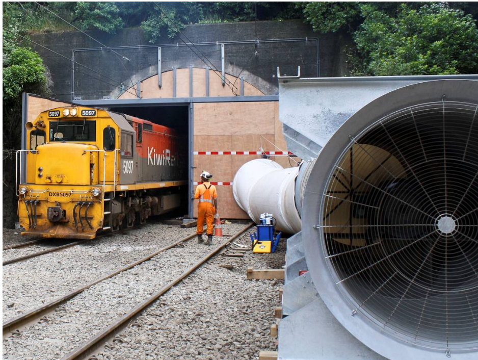
Tunnel 2 ventilation fan and door in use during Christmas block of line
