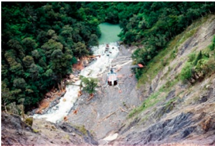
Figure 21: Landslip in gorge during 1982 flood – GWRC.
